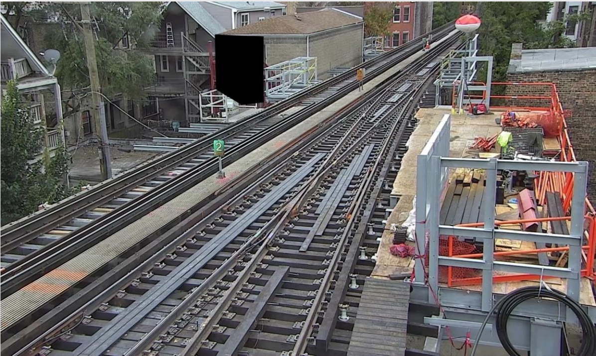
New interlocking, facing west
