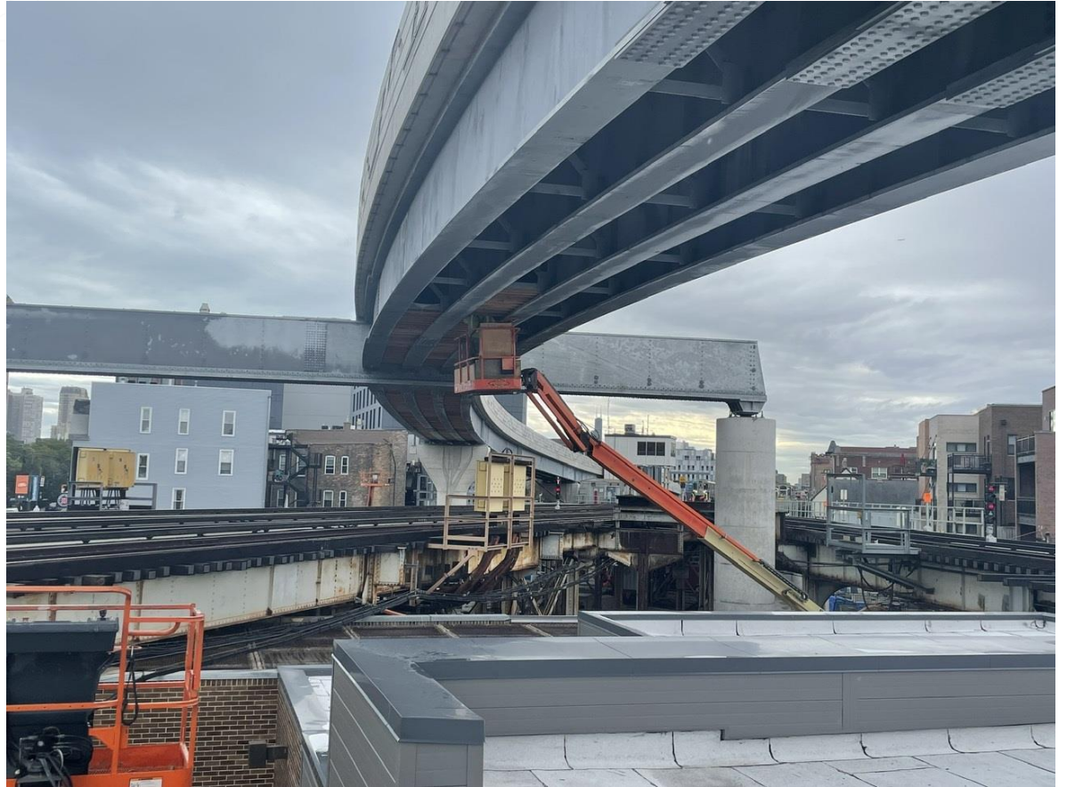
Looking southeast, Kimball-bound Brown Line trains will travel on the new bypass, above, crossing over Red and Purple Line tracks.
